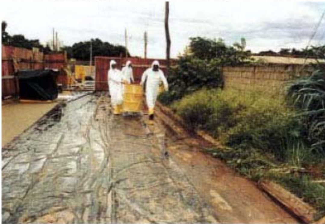
21. Much of the decontamination work had to be done in heavy rain.
