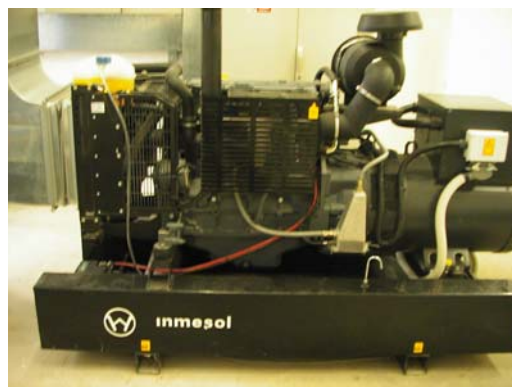
Obr.č.66 - Diesel agregát 65kWh
