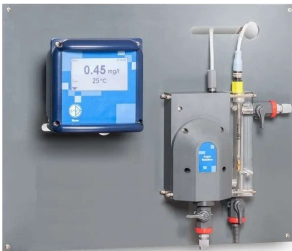
Obr. 4: Nalco Water Oxidant Controller [13]
